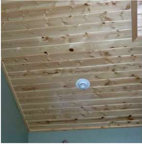
Recessed lights and unsealed wall ceiling junction.
