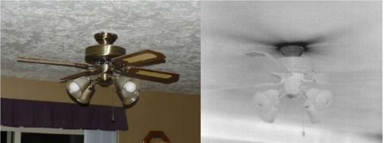
Left: air leakage at a ceiling fan. Right: IR picture of air leakage taken with blower door operating.
