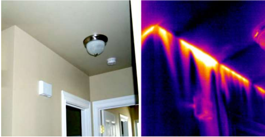
Top plate air leakage (hot attic).
