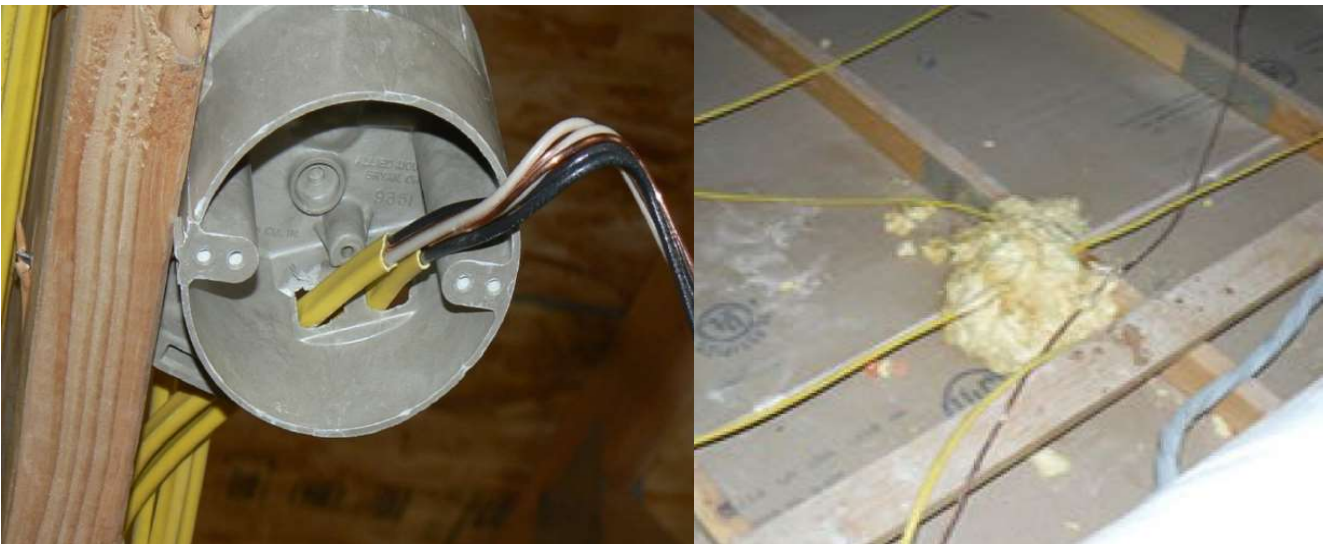
Standard ceiling electrical box with openings at wires and gaps between box and sheetrock (left). Fix: standard electrical box sealed with spray foam from attic (above right).
