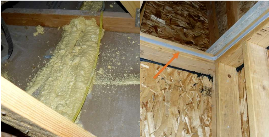
Fix: spray foam opening from the attic (left). Fix: top plate gasket sealing gap between sheetrock and top plate (right).
