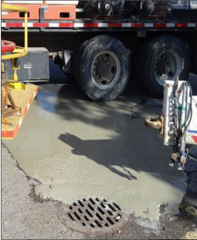
Graphic 4.0.1: Bentonite slurry spill
