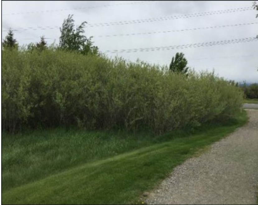
Image 6.0.1 Overgrown stormwater basin
