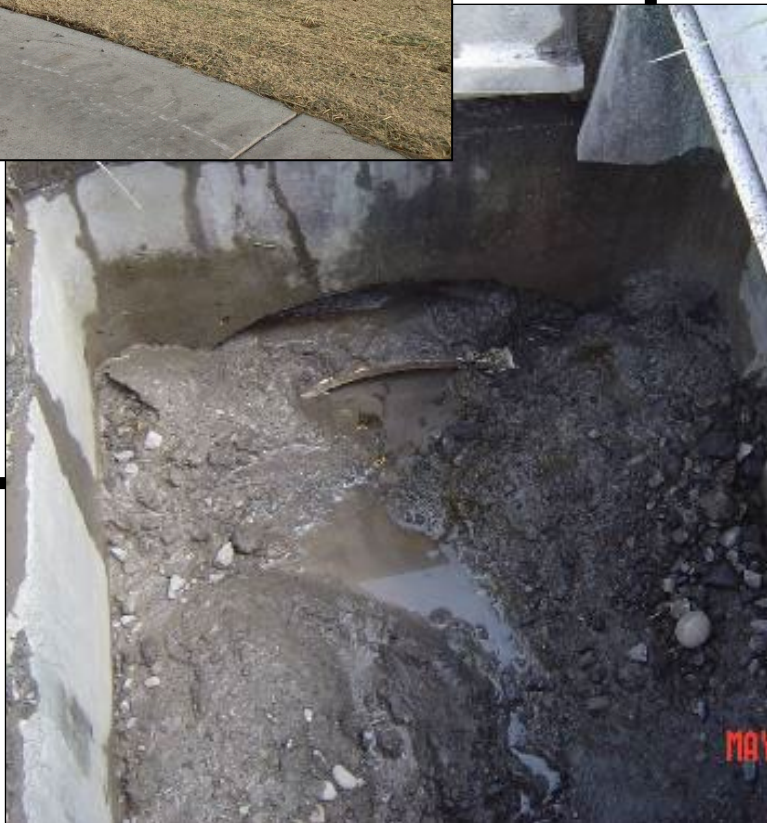
Graphic 5.0.2: Inlet sump clogged with construction debris
