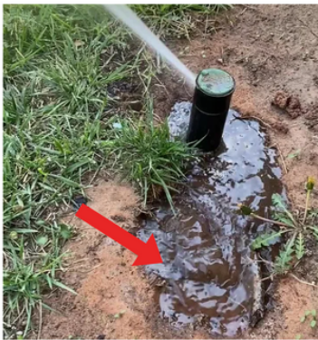
Pooling water at the base of the head often indicates a leak.
