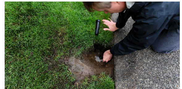
Excavation of the sprinkler head is often required to identify the source of the leak.
