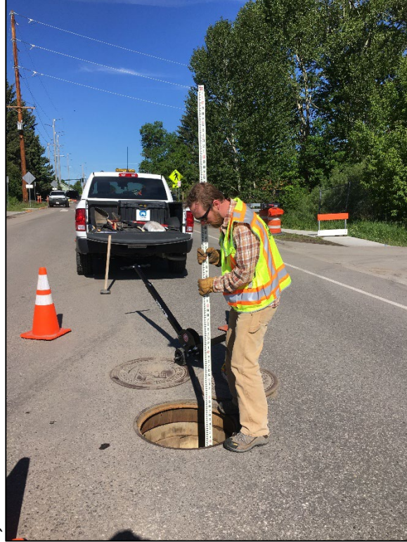
Figure 9 – Treatment Unit Debris Inspection and Measurement
