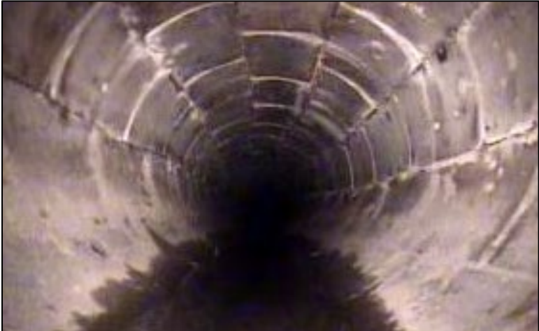
Figure 15 — Downtown VCP Pipe Condition
