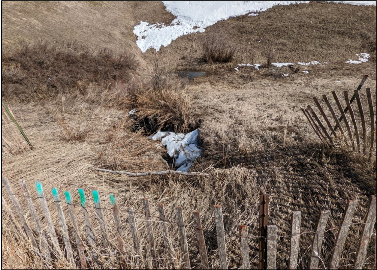
Figure 20 – Erosion at a Stormwater Outfall
