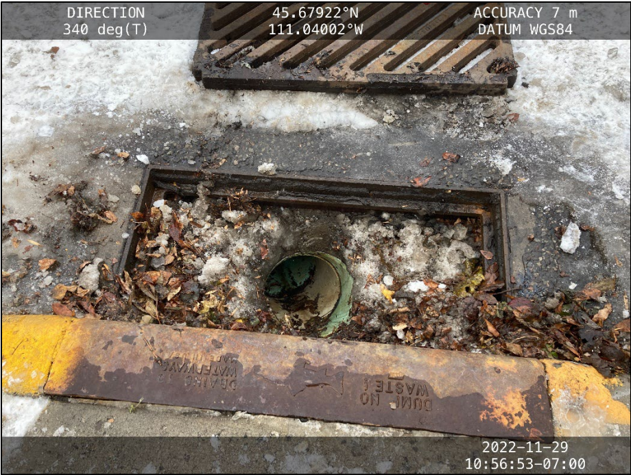
Figure 16 – Undersized Storm Drain Lateral on Main and Grand
