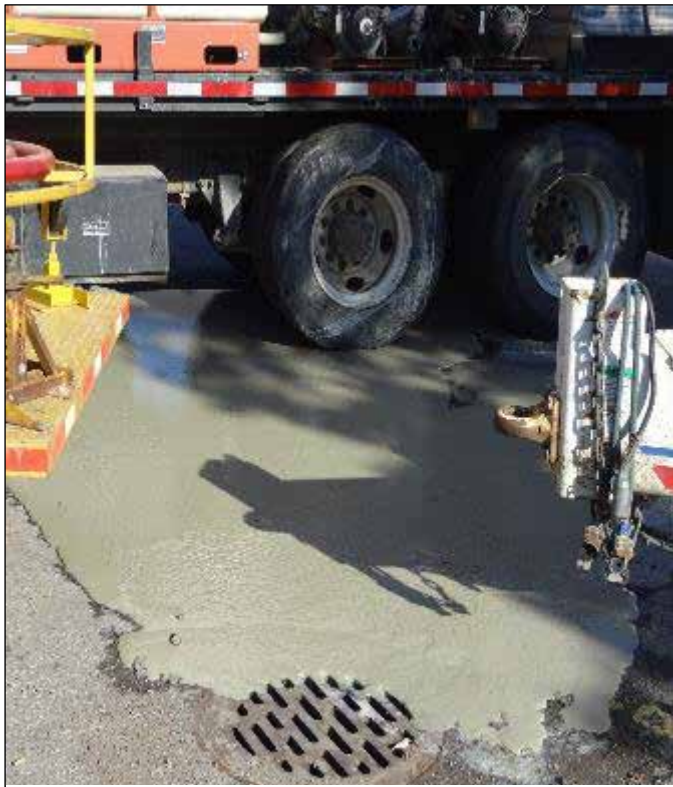
Graphic 4.0.1: Bentonite slurry spill
