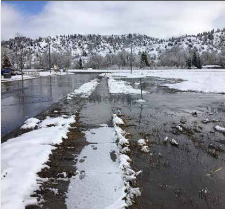
Graphic 1.0.1: Street flooding resulting from clogged
