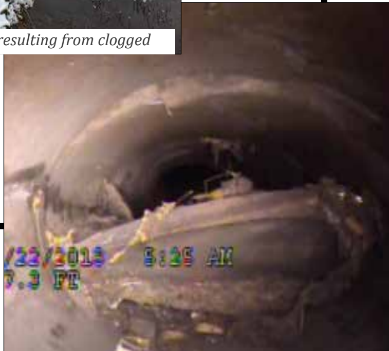
Graphic 1.0.2: Failed stormwater pipe
