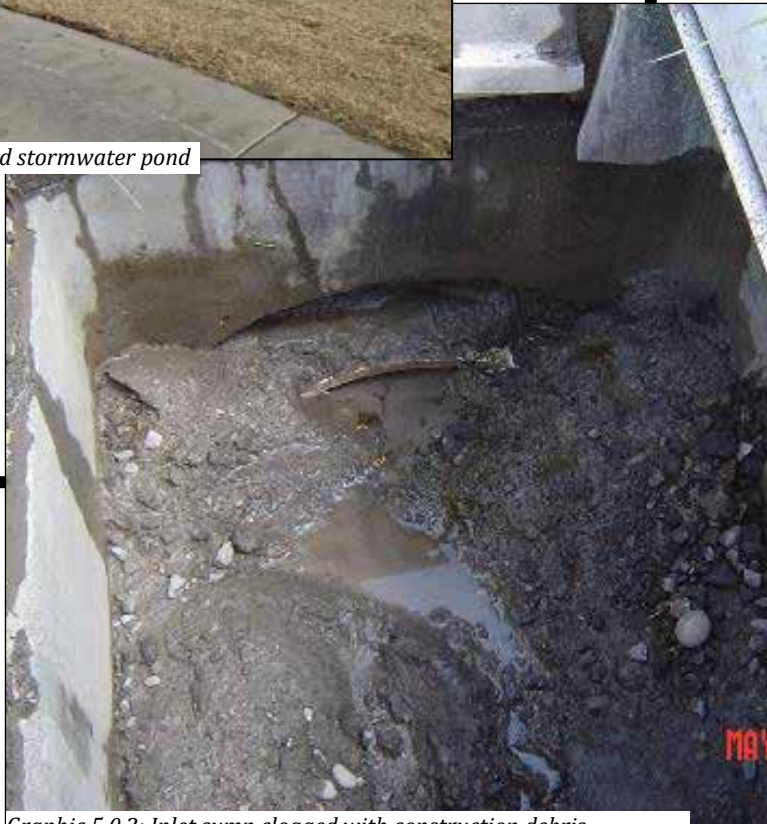
Graphic 5.0.2: Inlet sump clogged with construction debris
