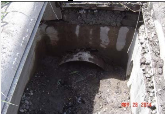
Image 3 - Clogged stormwater inlet from construction
