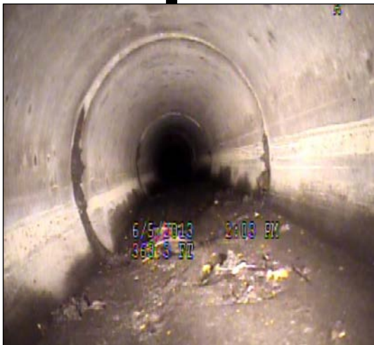
Image 1 - Clogged stormwater pipe from construction
