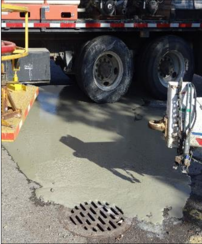
Image 4.0.1: Bentonite slurry spill
