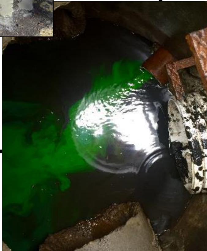
Image 4.0.2: Illicit connection confirmation through dye test
