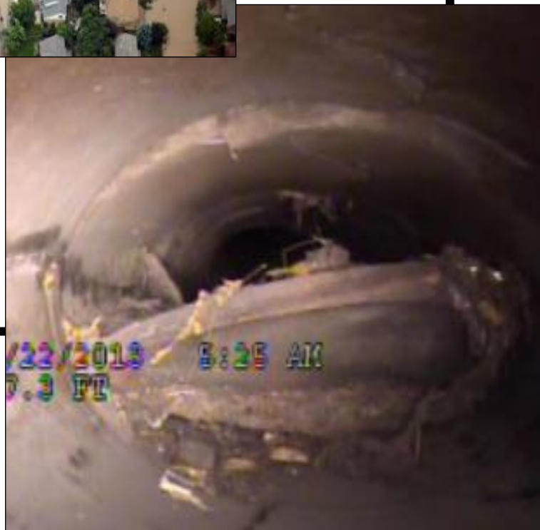
Image 1.0.2: Failed stormwater pipe
