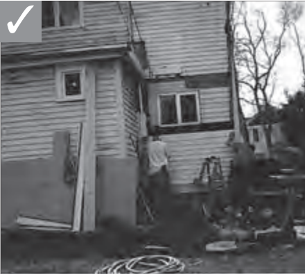
Repair wood features by patching or piecing-in new wood elements that match the original.
