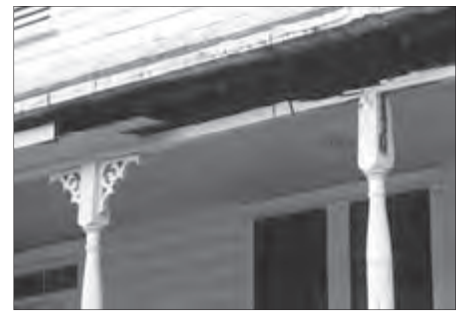
Replace missing original details in kind.
