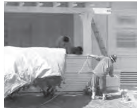
Protect wood siding and other wood surfaces with a painted finish.
